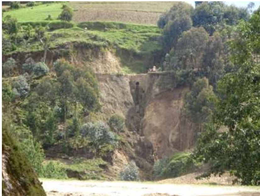
Figure 12: Erosion downstream of culvert in Sebeya catchment.
