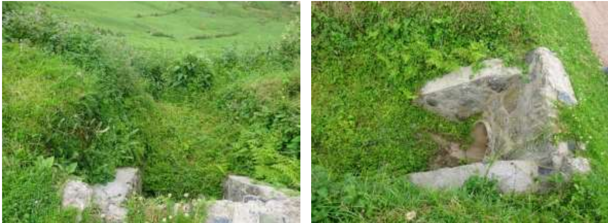
Figure 21: Grass vegetation at the culvert outlet protects the roadside environment from road-induced erosion.
