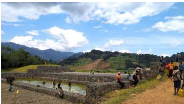
Figure 18: Dyke in Sebeya catchment. The construction of this dyke is part of the 'Embedding Integrated Water Resource Management in Rwanda (EWMR)' Project funded by the Embassy of the Kingdom of the Netherlands in Rwanda.
