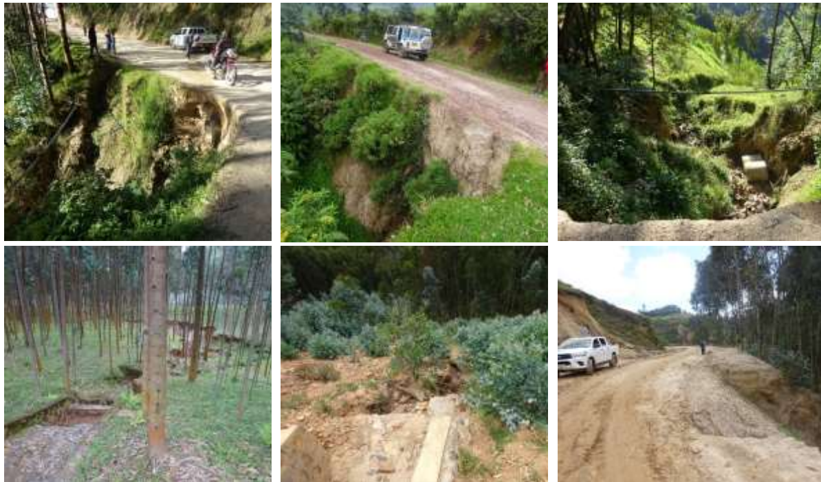
Figure 17: Road runoff causing erosion downstream of the culverts in Sebeya catchment.
