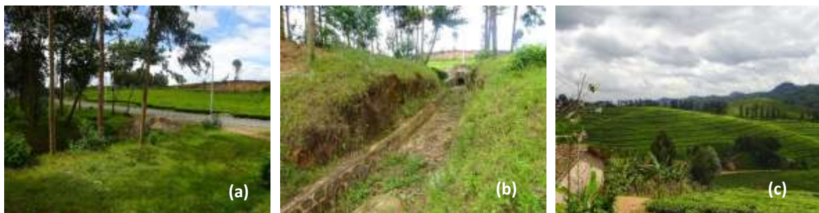
Figure 16: Masonry drains constructed at the culvert outlet to divert road runoff to tea plantations downstream of the road in Sebeya catchment (a) Road runoff collected from tarmac road, (b) Masonry water way constructed at culvert outlet, (c) Tea plantation benefiting of road runoff.
