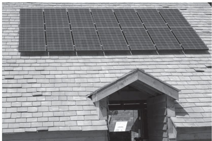
Picture 2. Every building can be a power station (Courtesy Nigel Dudley, Equilibrium Research)
