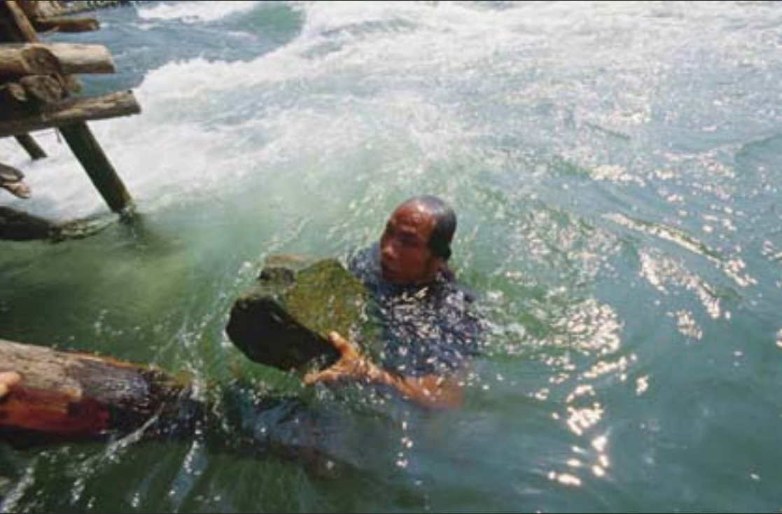
(Above) - Samnieng Khamphai continues the tradition of building a fall-back trap, taught to him by his father and grandfather before him. Only a few people use this dangerous technique. (Below) - Villagers dive to collect large stones to strengthen the foundations of their LI .
